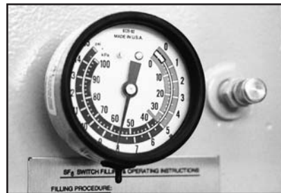
▲ Pressure gauge and fill valve
