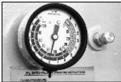
▲ Pressure gauge and fill valve
