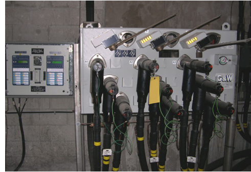
Vault switch with SEL controls.
