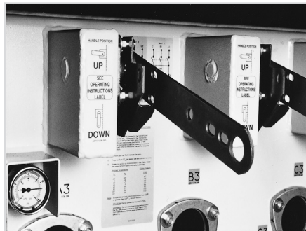
Single phase interrupter operating handles
