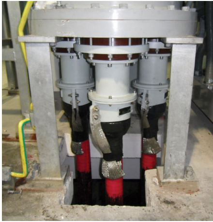
SSC140-SF terminations installed in a GIS.
