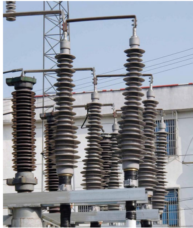
Dry type outdoor termination in a substation application.
