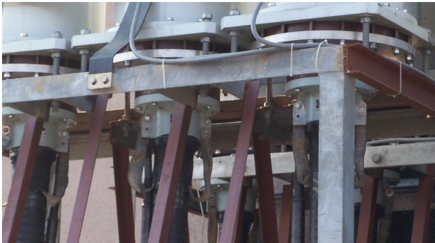
PATR140-SF terminations installed in a GIS.
