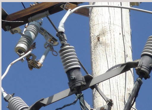
Distribution Cable Terminations
