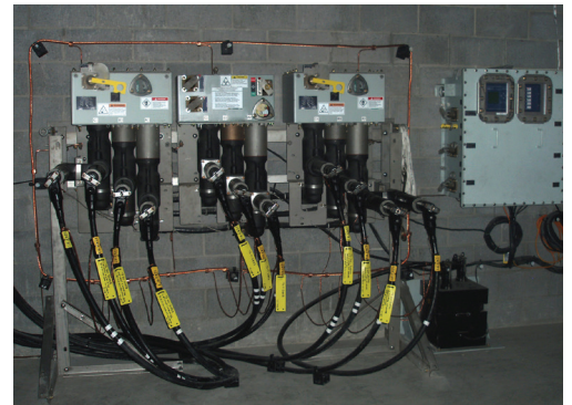
Solid Dielectric Vault
