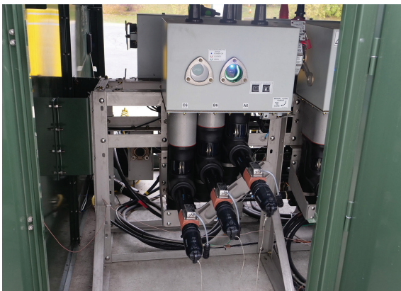
Underground platform with product installed (VS-27-UG)
