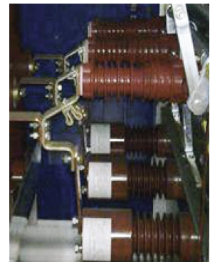
Voltage Sensor (VS-24-I – top) & Current Voltage Sensor (CVS-24-I – bottom) installed in switchgear application
