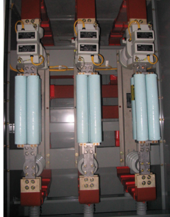
CLiP used in a large offshore deepwater oil platform
