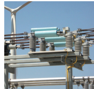
CLiP protecting the substation of a midwestern windfarm
