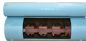
Close up of the severed main conductor and melted current limiting element of a 3000A (double bus) CLiP after interruption
